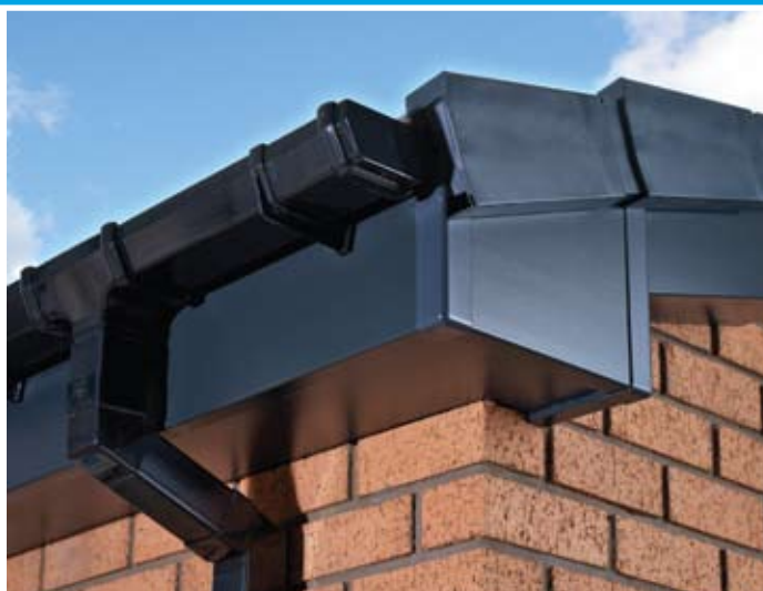
Dark Grey Fascia Black Square Rainwater
